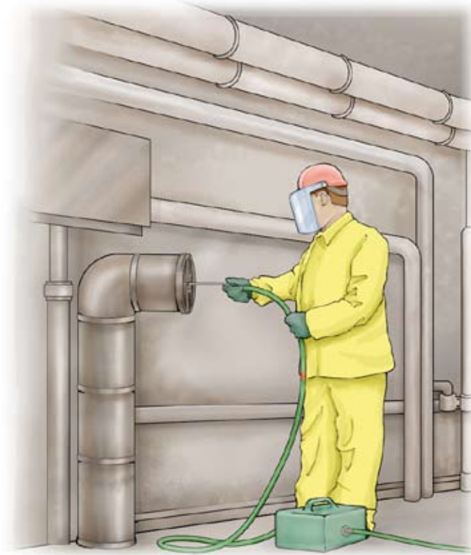
Figure 22. Work should be done between foot and shoulder height, as it is difficult to control the flex-lance if it is higher than the shoulder.
